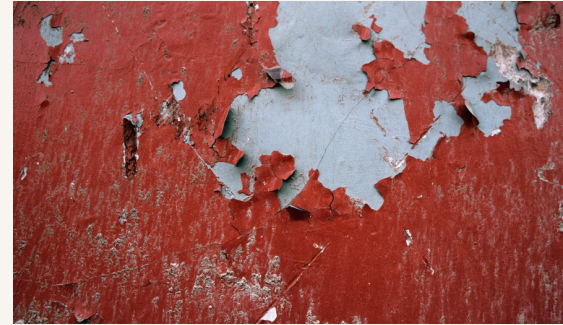
Paints flakes off a metal surface. Image source: Alamy
